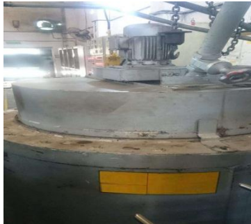
PIT TYPE FURNACE (650°C)
